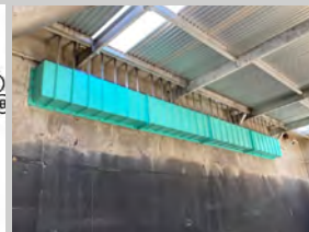
Inboard weirs provide flow splitting and increased the sidewater depth to reduce energy costs
