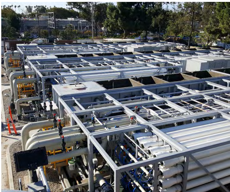
Exhibit 6-9 / IDE and Kiewit utilized preassembled modules to deliver quality, save time and reduce installation costs on this fast-tracked project.
