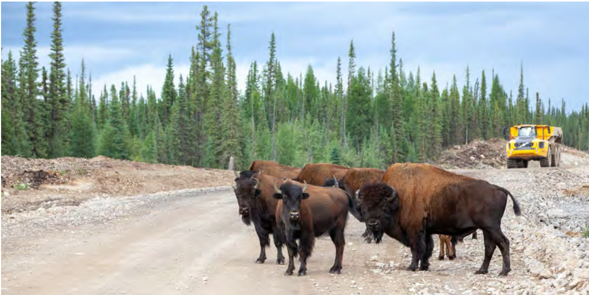
Exhibit 5-5 / Kiewit Development helped secure the Tłı̄chǫ All-Season Road project funding with the Government of Canada (25%) and the Government of the Northwest Territories (75%) to serve the First Nations (indigenous people) communities in subarctic Whati.
