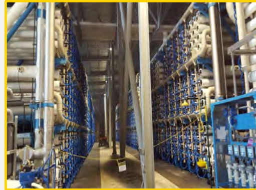
Exhibit 3-4 / Claude Bud Lewis Carlsbad Desalination Plant PDB
