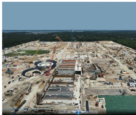
Northeast Water Purification Plant City of Houston
