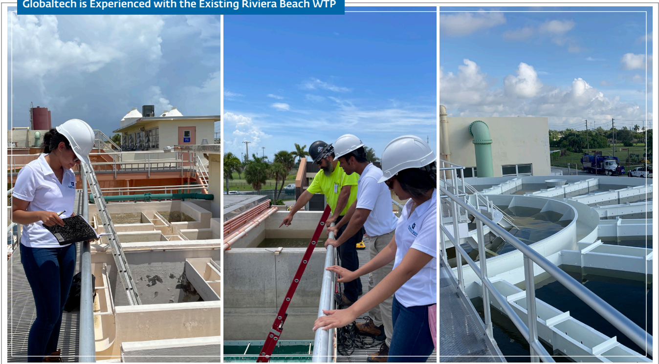
Globaltech is Experienced with the Existing Riviera Beach WTP
