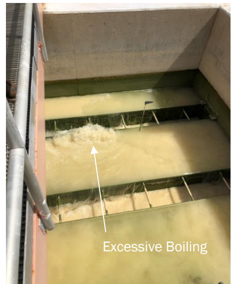
Figure 4-3. Nonuniform Backwash flow Observed (Filter #14)
