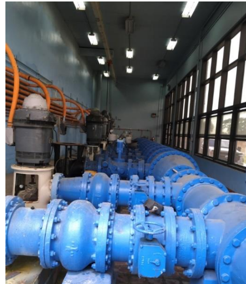
Figure 4-11. Transfer Pumps and Piping Discharge Missing ARVs
