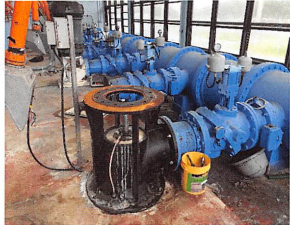
Figure 3. No visible grout on HSP No. 1
