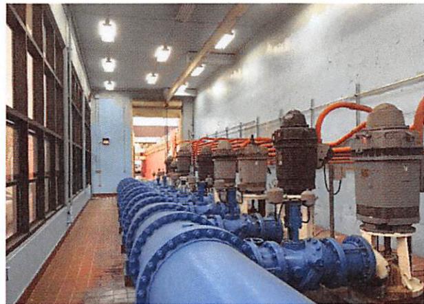
Figure 1. Existing High Service Pumps
