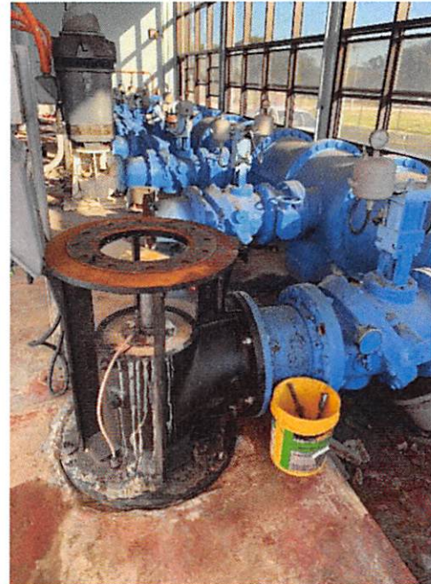
Figure 7. No sole plate on newly installed pump
