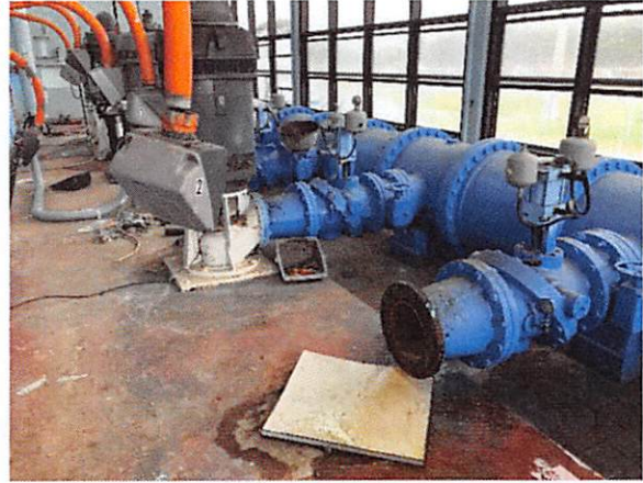
Figure 11. Exposed floor penetration not secured properly for HSP No. 2
