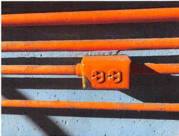
Figure 12. Open electrical outlet
