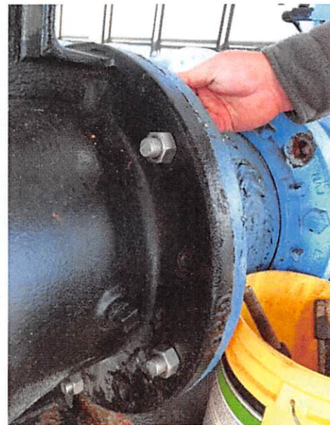
Figure 9. Missing bolts on pump flange
