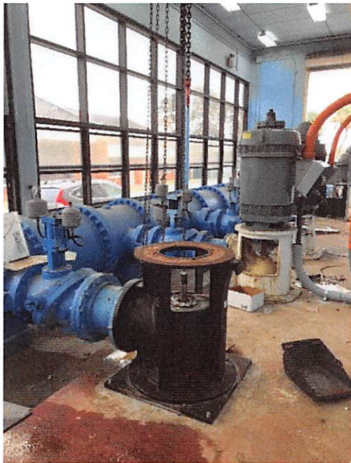
Figure 6. No shaft guards on any pump
