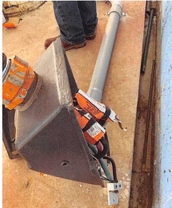
Figure 13. Exposed electric wires
