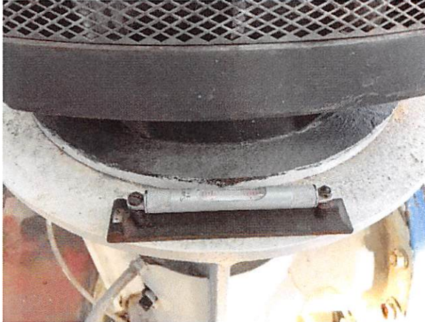
Figure 2. Uneven level of an installed pump
