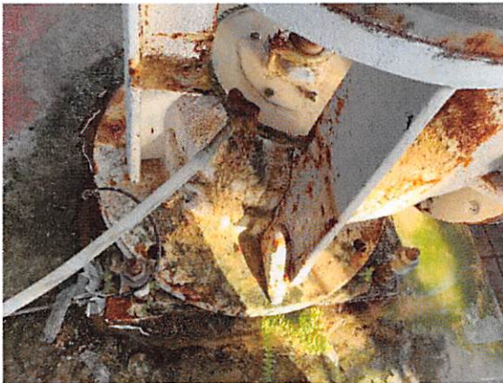
Figure 8. Missing bolts and constant seal water flow at HSP No. 7
