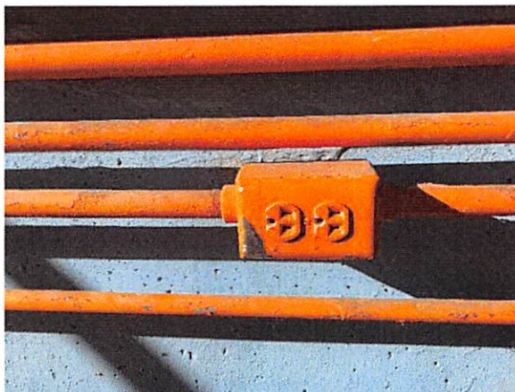
Figure 12. Open electrical outlet
