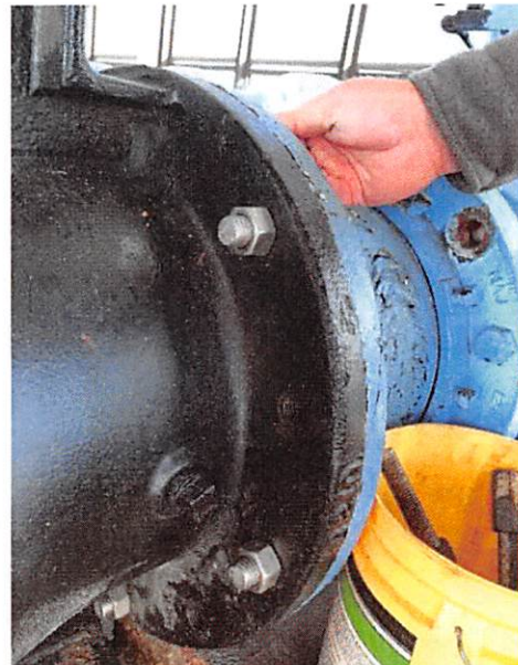
Figure 9. Missing bolts on pump flange
