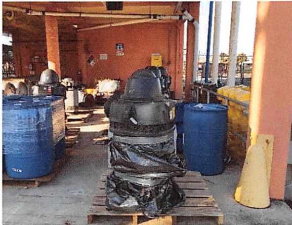
Figure 10. New uninstalled HSP motors
