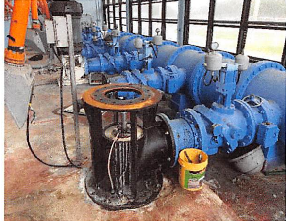
Figure 3. No visible grout on HSP No. 1
