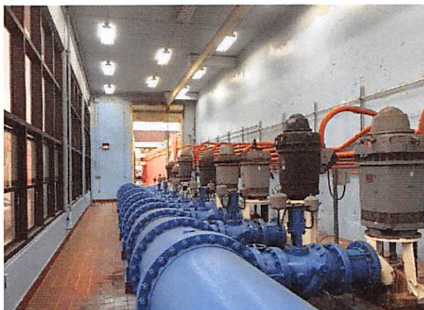
Figure 1. Existing High Service Pumps
