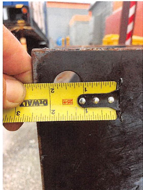
Figure 5. Sole plate bolt holes of uninstalled pumps
