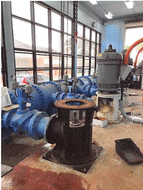
Figure 6. No shaft guards on any pump
