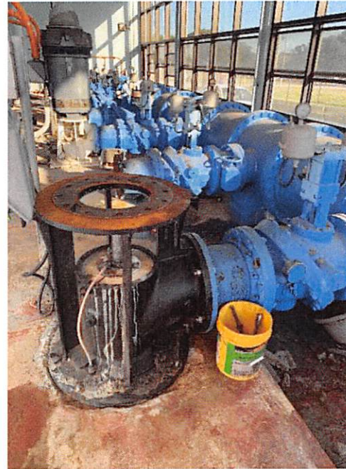
Figure 7. No sole plate on newly installed pump
