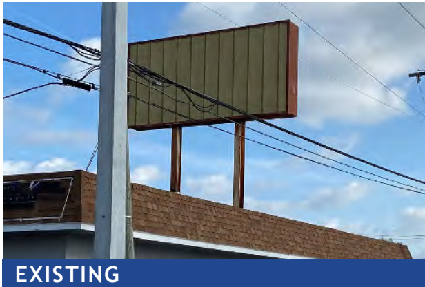
Figure 2 Image of empty sign which does not meet existing code.
