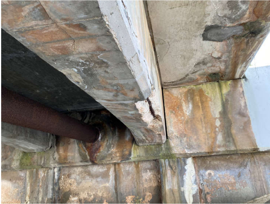
Photo 13: Island Drive – SW Bridge Outer Beam North Side
