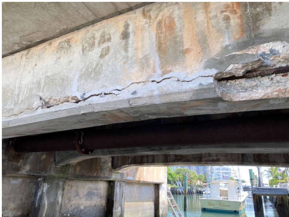
Photo 10: Island Drive – SW Bridge Outer Beam North Side
