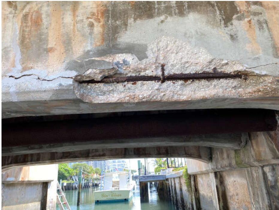
Photo 9: Island Drive – SW Bridge Outer Beam North Side
