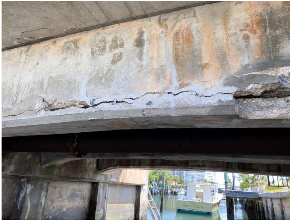
Photo 11: Island Drive – SW Bridge Outer Beam North Side
