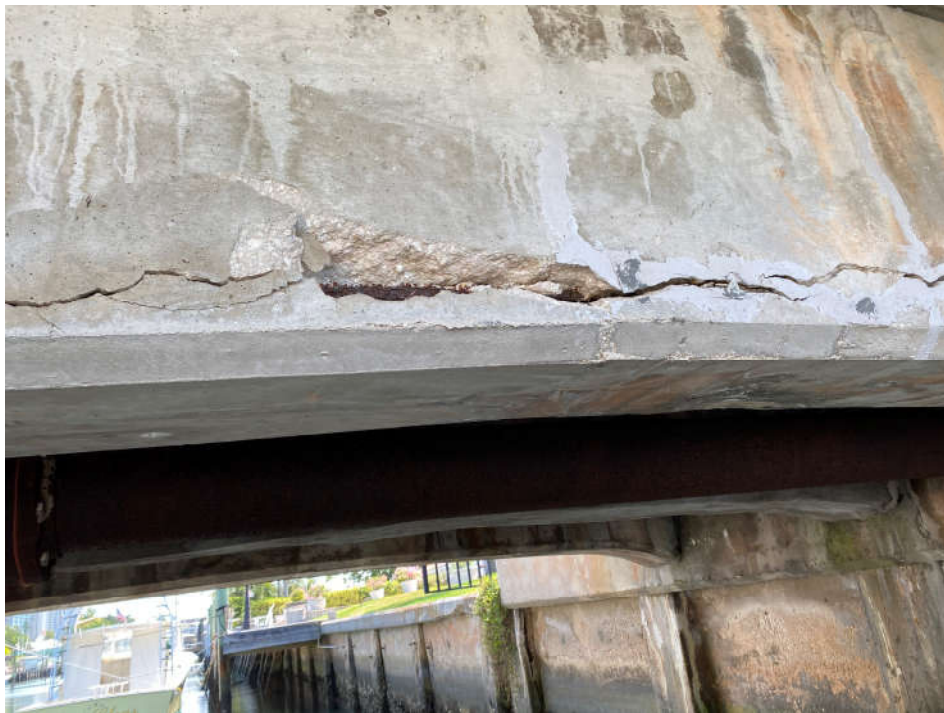
Photo 12: Island Drive – SW Bridge Outer Beam North Side
