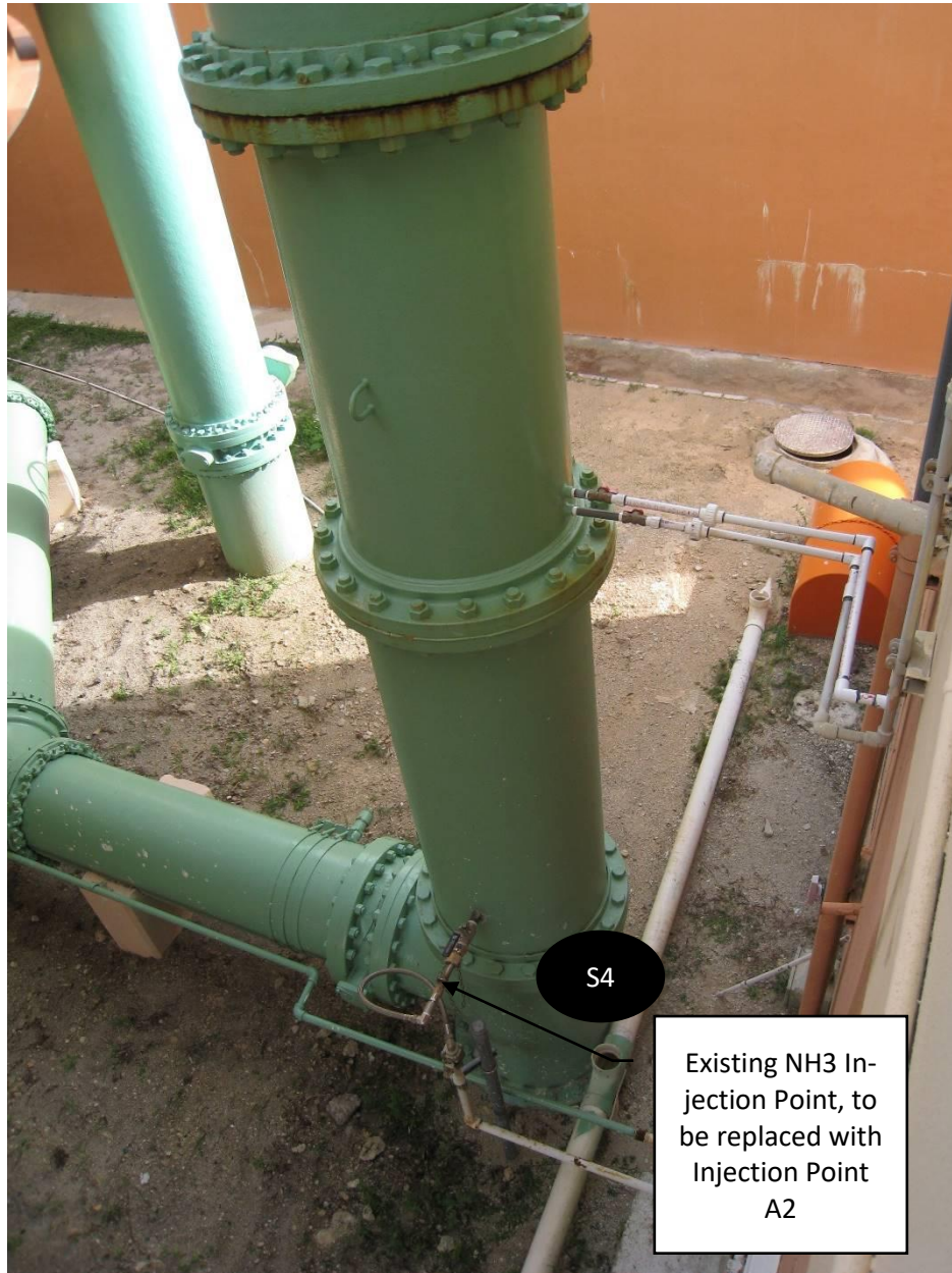
Figure A-4. Influent Pipe to South Chemical Building Influent Basin
