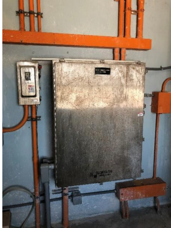
Figure 6-2. PLCs in North Chemical Building on South Wall
