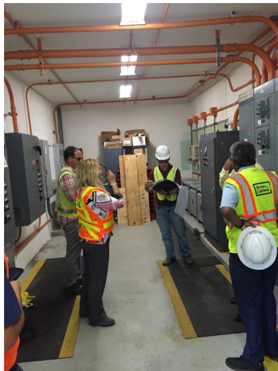
Figure 6-3. Interior of air stripper electrical room during 2019 Site Visit
