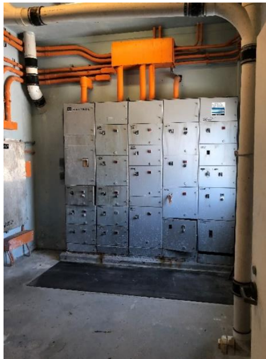
Figure 6-1. MCC-3 in poor condition on West Wall
