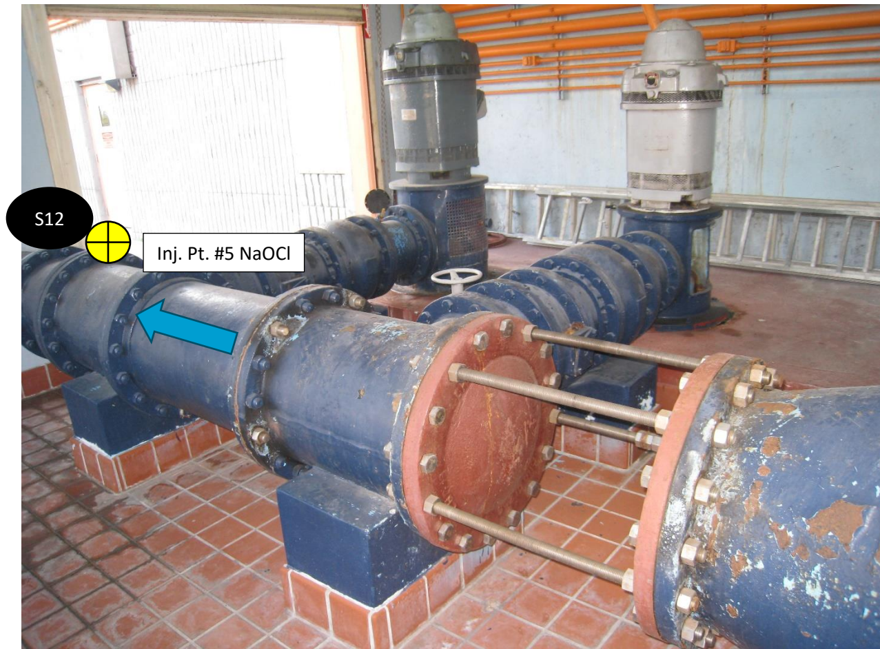
Figure A-10. Transfer and Backwash Pumps (South end of High Service Pump Room)
