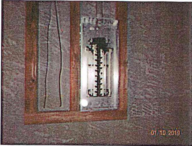
Electrical Panel - East Interior Wall
