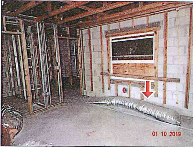
Damaged AC duct
