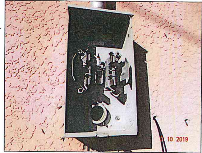
Electrical Panel - East Wall
