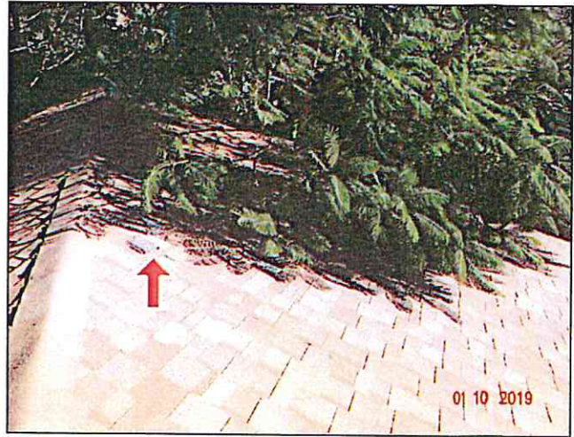
Damaged Roof Shingle
