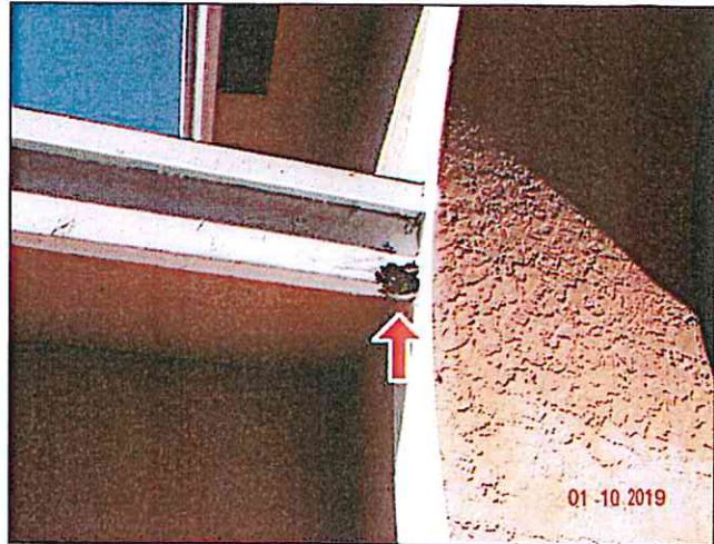
Wood Rot - West Fascia
