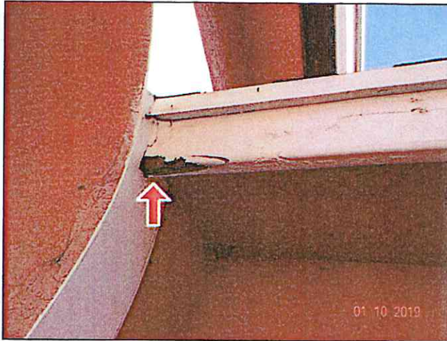
Wood Rot - East Fascia
