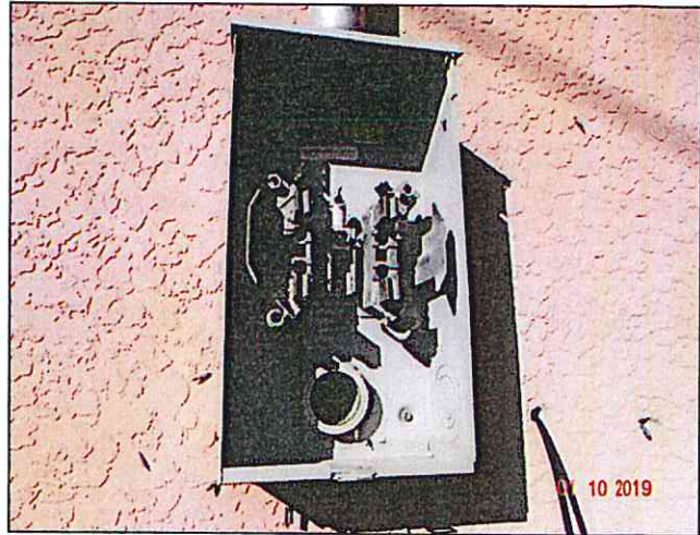
Electrical Panel - East Wall
