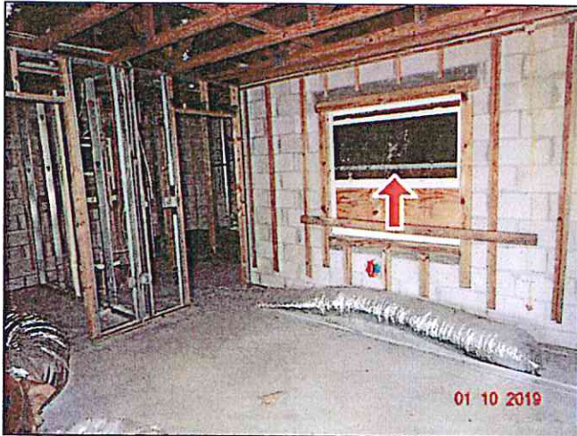
Damaged Window - Master Bedroom
