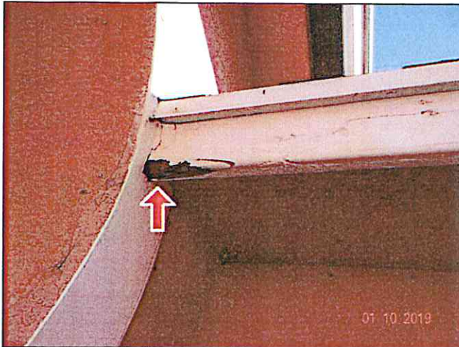
Wood Rot - East Fascia
