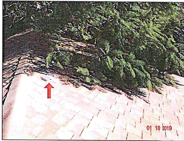
Damaged Roof Shingle
