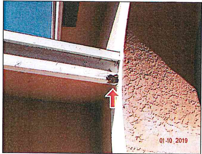
Wood Rot - West Fascia
