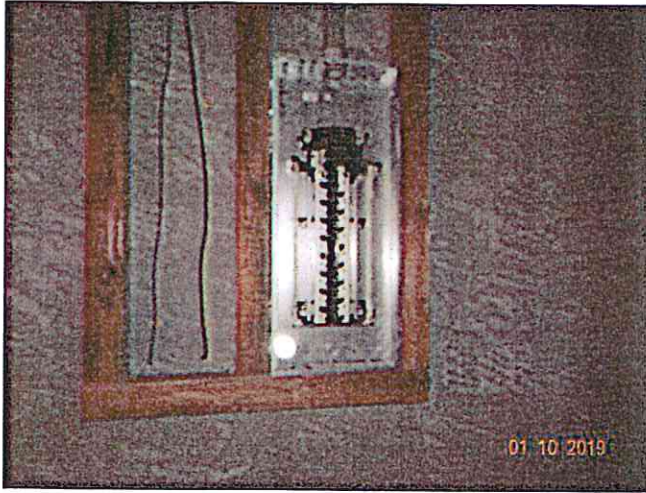
Electrical Panel - East Interior Wall
