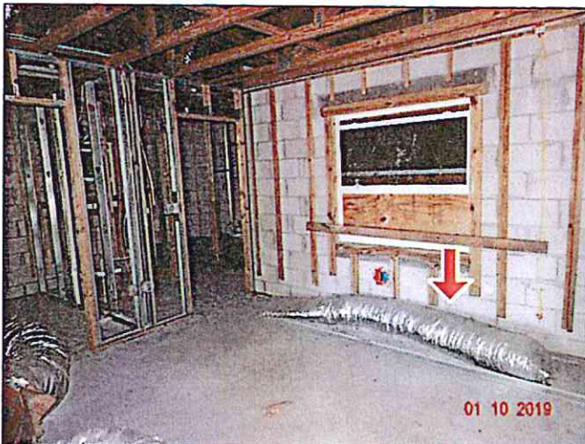
Damaged AC duct
