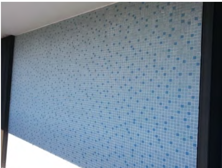
48. View of mosaic tile wall finish noted on the south side of the building.
