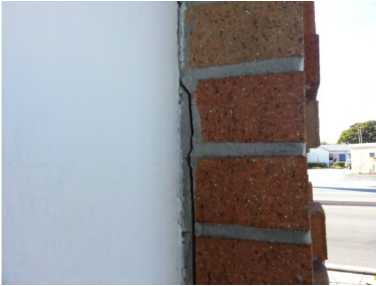
37. View of cracked joint noted between the brick and concrete walls at the northeast corner of the northwest stairway.
