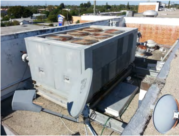
22. View of the packaged chiller unit noted on the lower roof area over the mechanical room.
