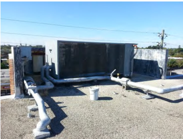
24. View of the 2 nd packaged chiller unit noted in the west portion of the north roof.
