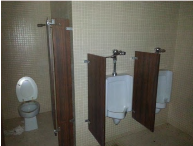
71. View of urinals and water closet noted in the men's toilet room in the west portion of the 2 nd floor.
