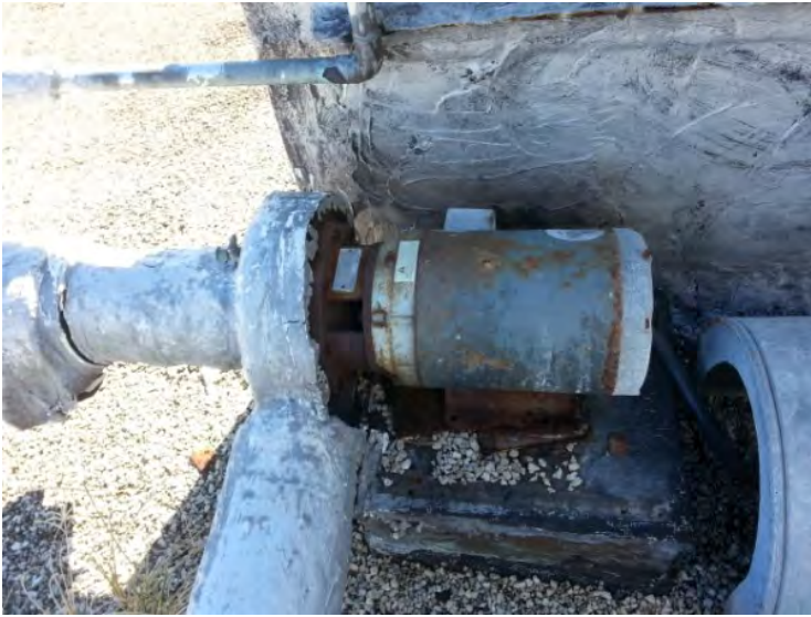
25. View of the chilled water pump noted near the 2 nd chiller unit.
