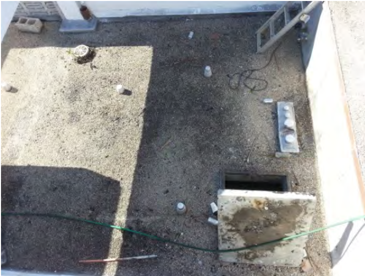
20. View of the roof access located over the lower roof of the mechanical room. Note the corrosion on the roof hatch.
