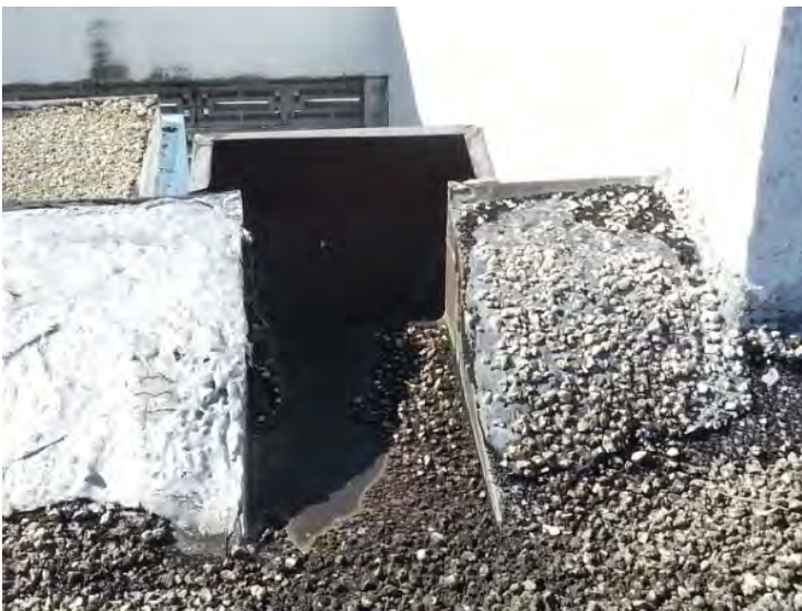
18. View of a roof drainage scupper noted at the west side of the south roof.
