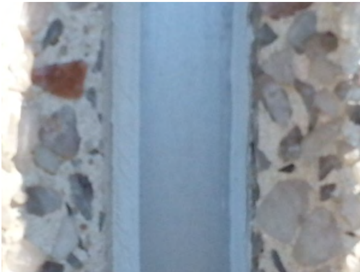
38. View of precast concrete wall joint detail noted on the west side of the building.
