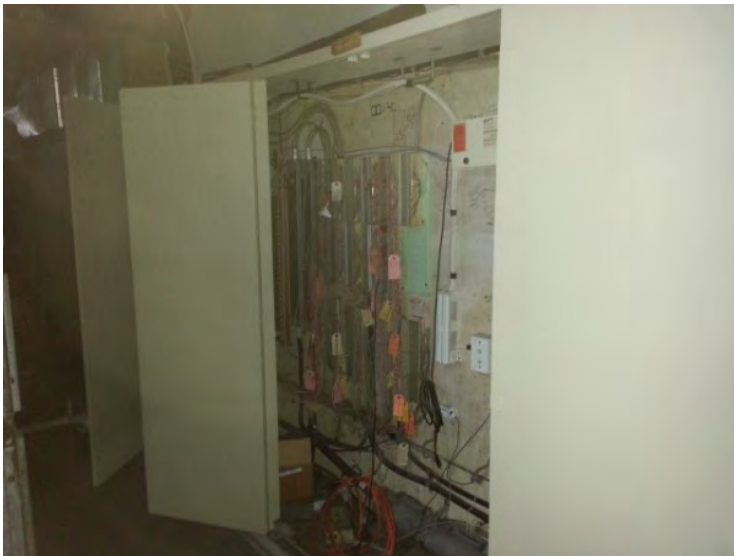
83. View of the telecom cabinet noted in the mechanical room in the west portion of the building.
