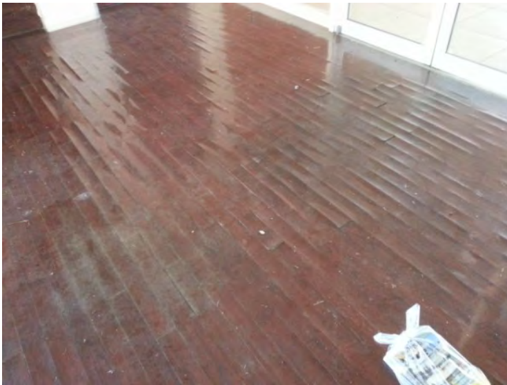
56. View of damaged wood flooring noted at the north entrance vestibule.
