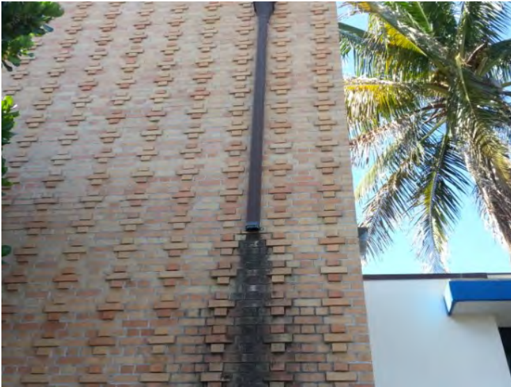
14. View of missing downspout noted on the east side of the building.
