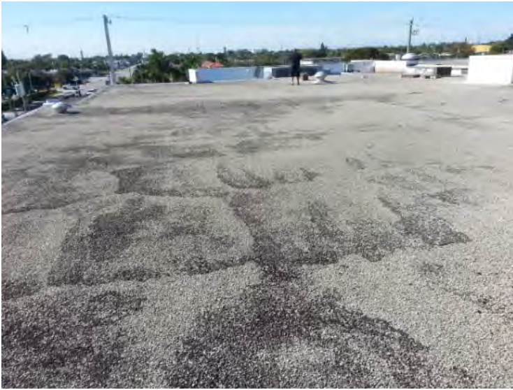
16. View looking west at the south roof of the building noting the condition.
