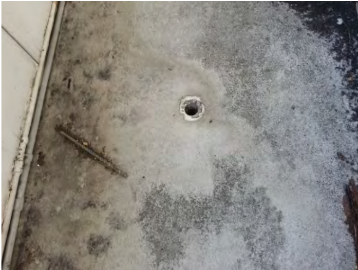
47. View of typical balcony floor drain with missing strainer cover noted at the south side of the building. Note the staining of the balcony floor.
