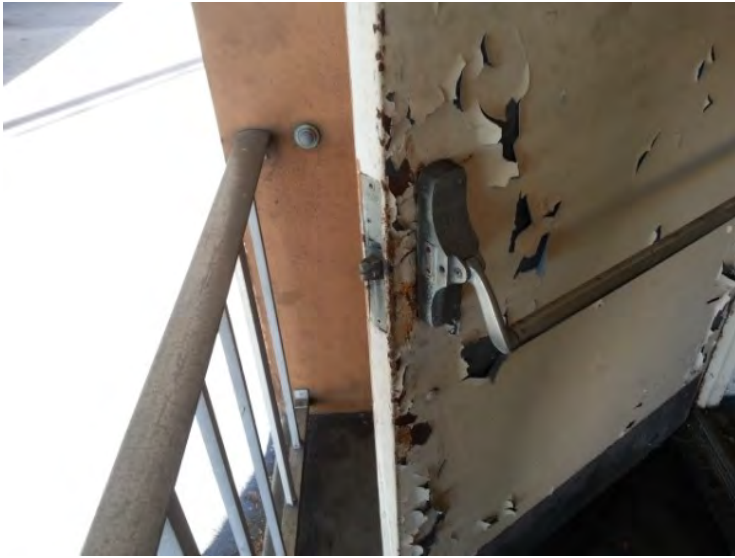
43. View of peeling paint and corroding metal surfaces noted on the exit door from the northwest stairway.
