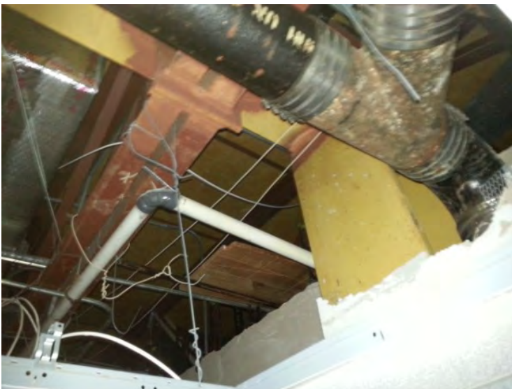
81. View of the structural steel framing of the building noted on the 2 nd floor.
