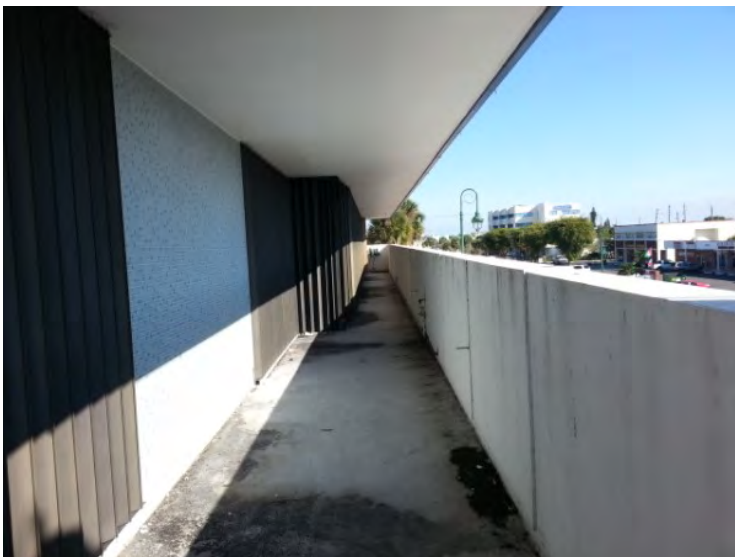
45. View looking east at the 2 nd floor balcony on the south side of the building.
