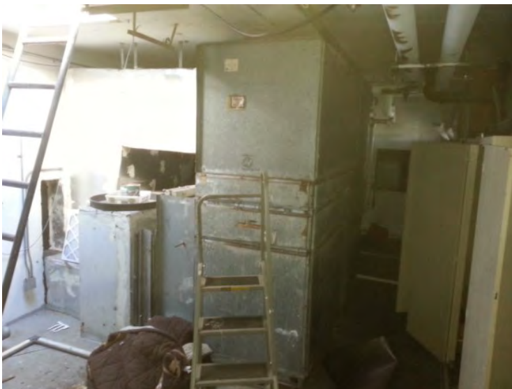
87. View of one of the two built-up air-handling unit noted in the mechanical room in the west portion of the building.
