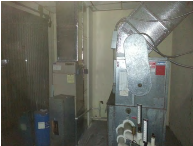
86. View of HVAC equipment noted in the north portion of the mechanical room.
