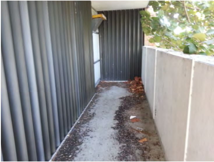
46. View of debris accumulation noted at the east side balcony on the 2 nd floor.
