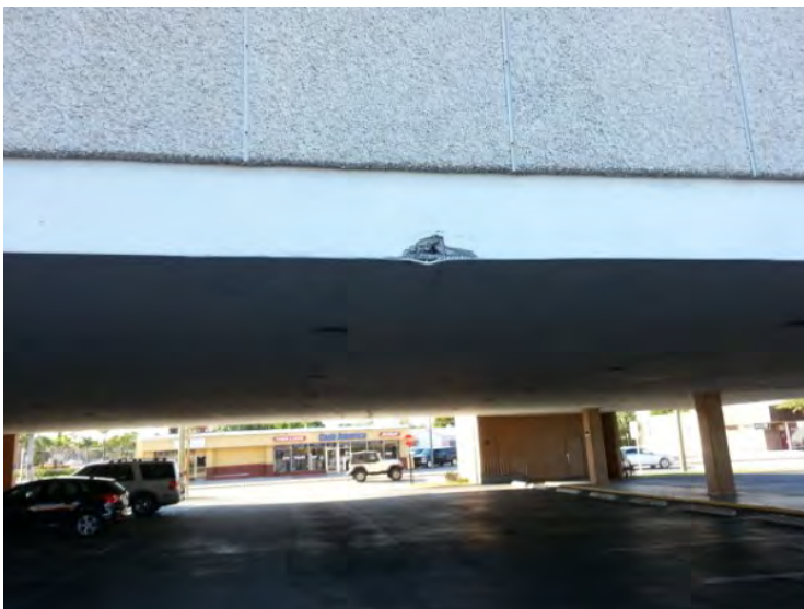
42. View of damaged soffit noted at the entrance header at the east side access to the covered parking spaces.
