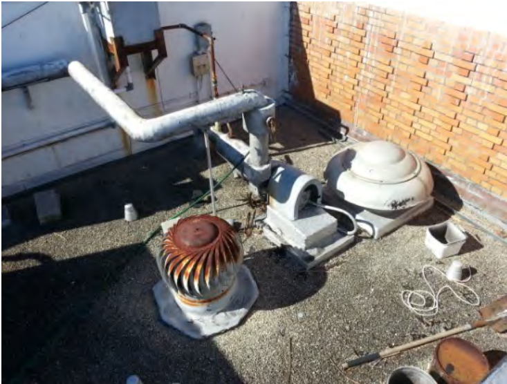
23. View of corroding exhaust fans and mechanical room turbine vent noted on the roof of the mechanical room in the west portion of the building.
