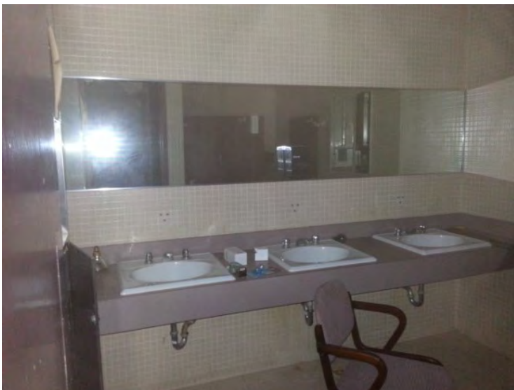
69. View of the lavatory in the women's toilet room located in the west portion of the 2 nd floor.
