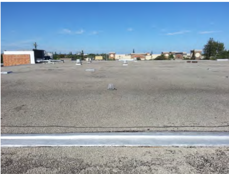
21. View looking north at the north roof area noting the membrane flashing over the expansion in the foreground.
