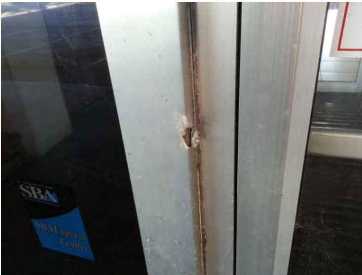
54. View of damaged storefront frame noted at the north entrance to the building.
