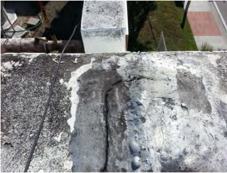
19. View of an open crack noted on the roof coping near the south packaged chiller area.
