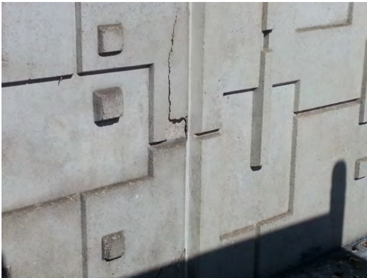
35. View of cracking noted on the patterned precast concrete wall at the south side of the building.
