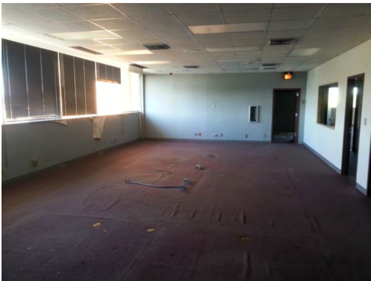
75. General view in the 2 nd floor office area. Note the condition of the vinyl wall covering and the flooring.
