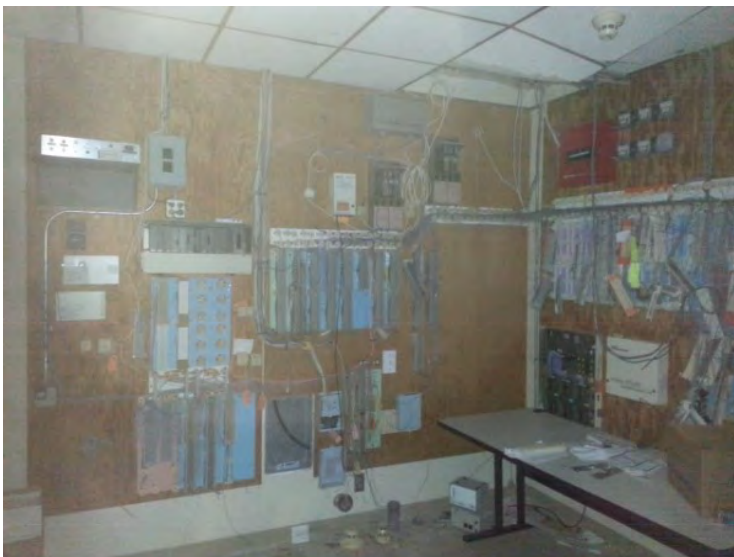
84. View in the telecom and computer room located on the 2 nd floor of the building.
