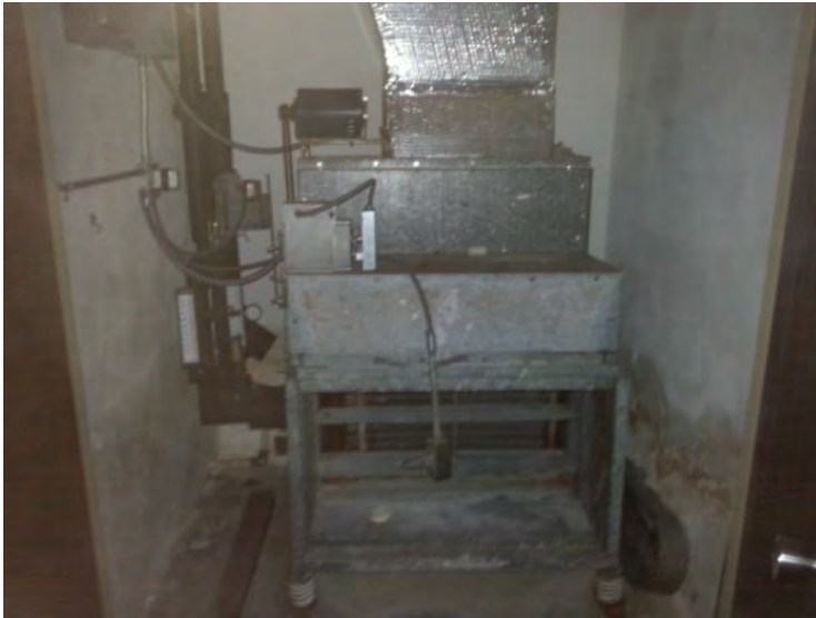
85. View of an HVAC equipment noted in the east portion of the 2 nd floor.
