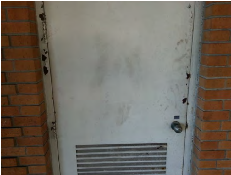
44. View of corroding metal door noted at the south side of the building.
