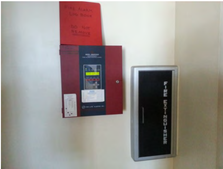
82. View of the fire alarm control panel noted in the north portion of the 1 st floor. Note the typical fire extinguisher.
