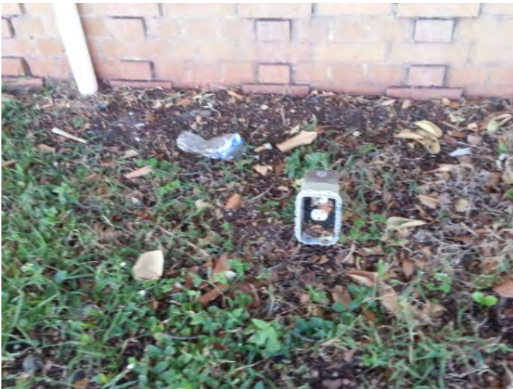
15. View of missing cover noted on an electric power receptacle at the east side of the building.
