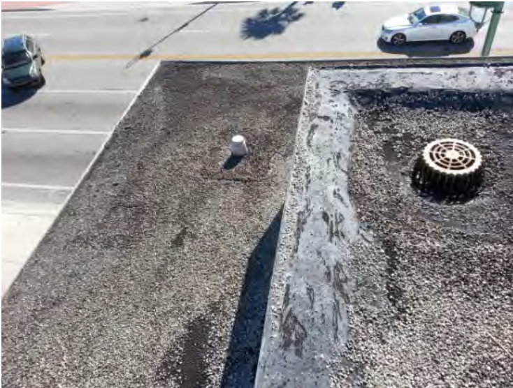
17. View at the southeast corner of the south roof noting the lower roof over the balcony and the interior drain on the main roof level.
