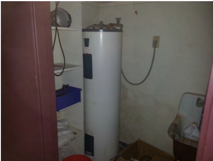
89. View of an electric water heater noted in the west portion of the 2 nd floor.
