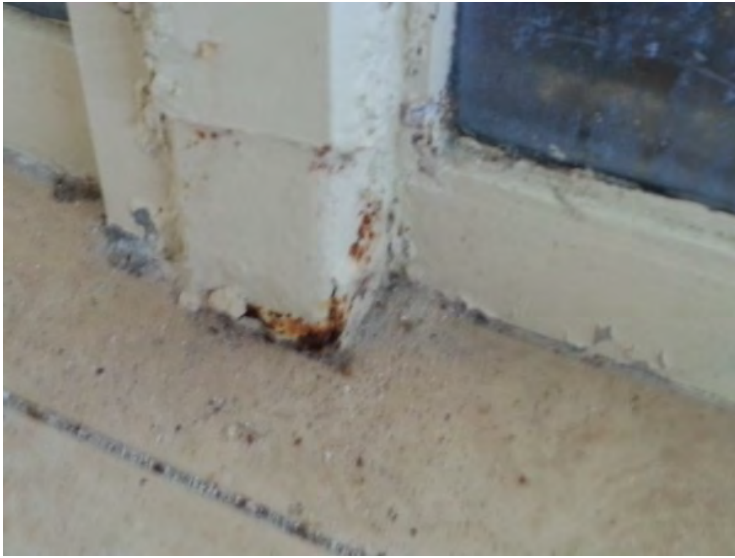
55. View of corroding storefront metal frame noted in the building at the east storefront assembly.
