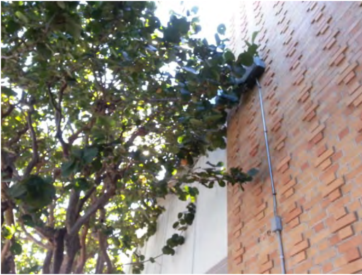
13. View of tree contact with the building noted on the east side.
