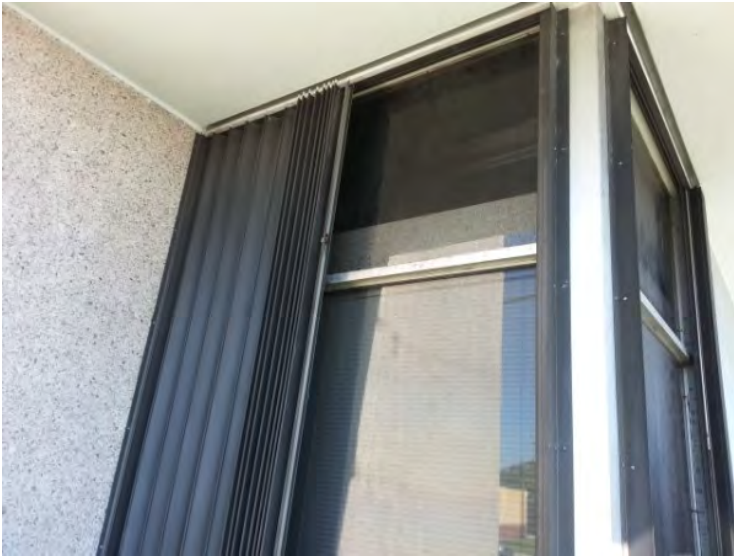
49. View of typical storefront assembly with hurricane shield noted on the building.
