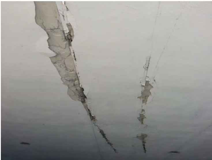
41. View of damaged soffit noted on the west-end portion of the carport.
