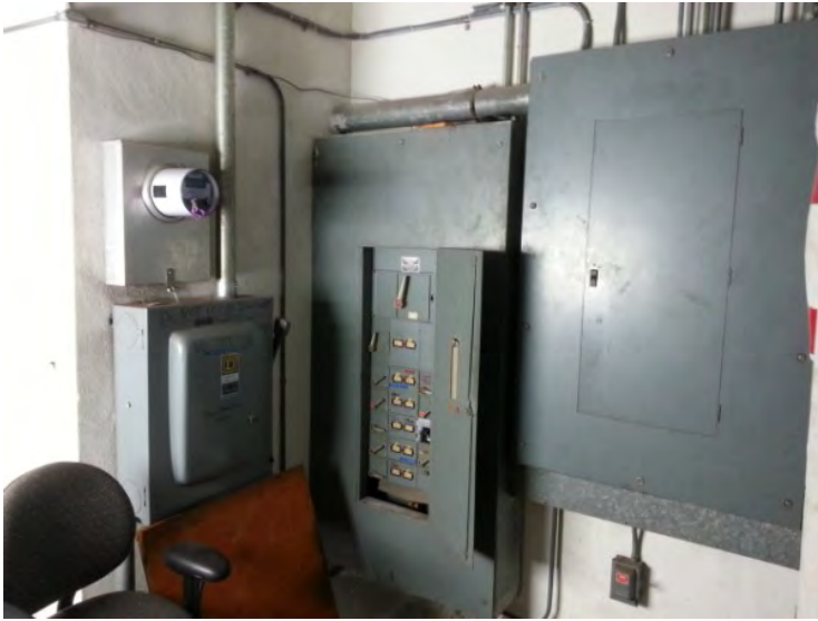
88. View of electrical main panel noted in the mechanical room in the west portion of the building.
