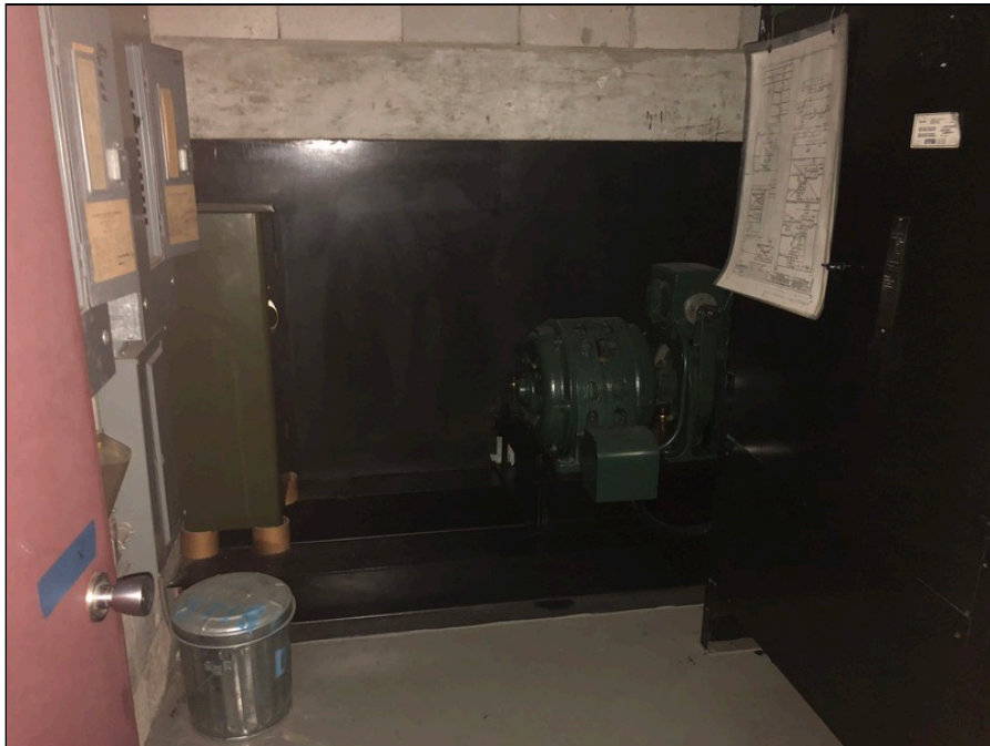
10 - View of elevator motor
