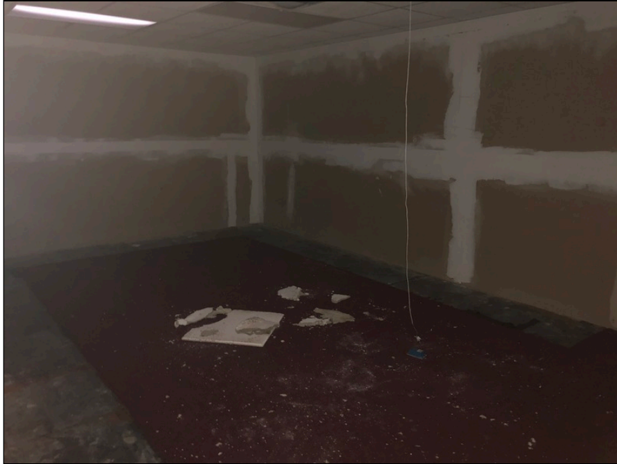
5 - Vacant office space in disrepair
