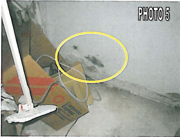
Police Department Room P244 – Suspect visible mold (SVM) on drywall in southeast corner.
