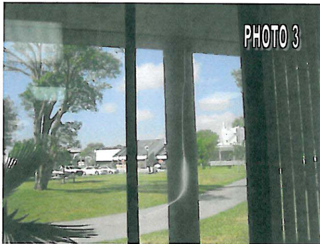
City Hall Room C115 - Crack in exterior window pane.
