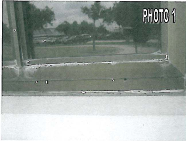
City Hall Exterior - Water stains and corrosion on window sill.
