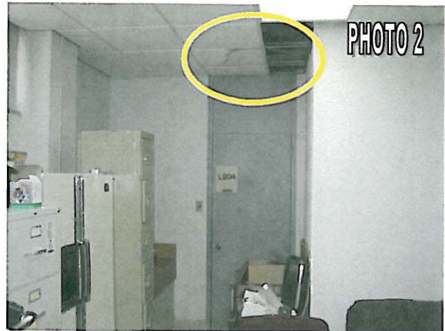
Library Staff Lounge - Stains on ceiling tiles and missing tiles.
