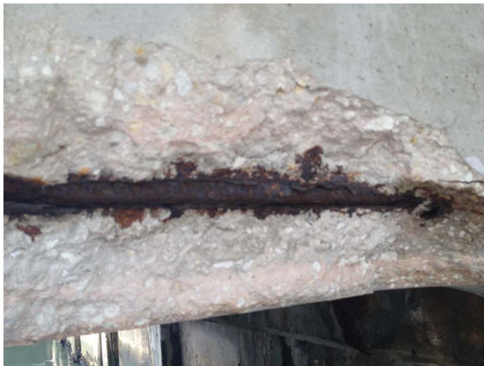
Figure 29: Reinforcing Corrosion Island Drive Structure
