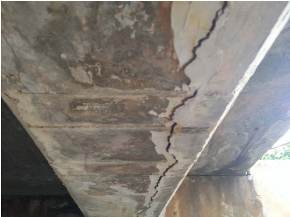
Figure 24: Beam Cracking Island Drive Structure
