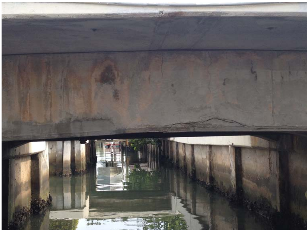
Figure 23: Beam Cracking Island Drive Structure
