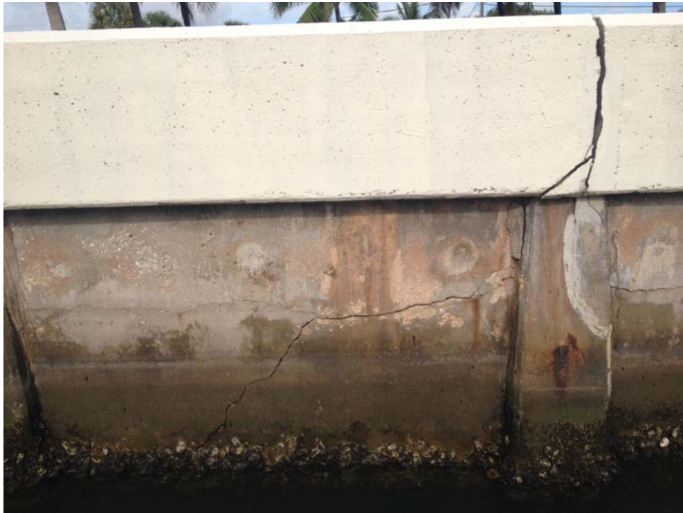
Figure 34: Bulkhead Cap & Sheet Panel Cracking Island Drive Structures
