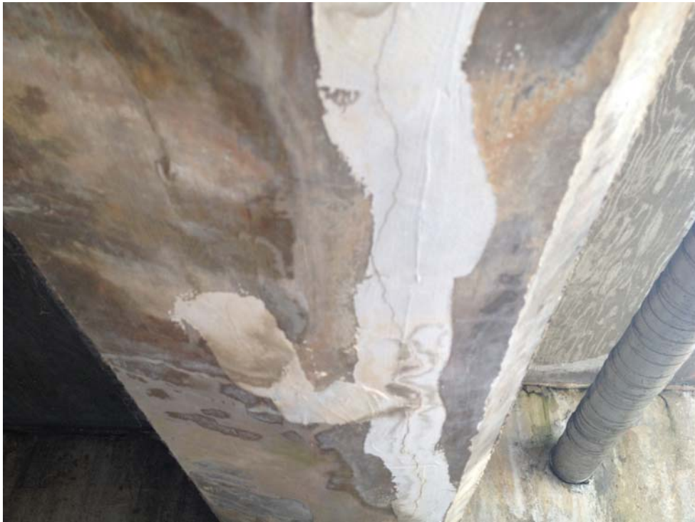
Figure 20: Beam Cracking Island Drive Structure
