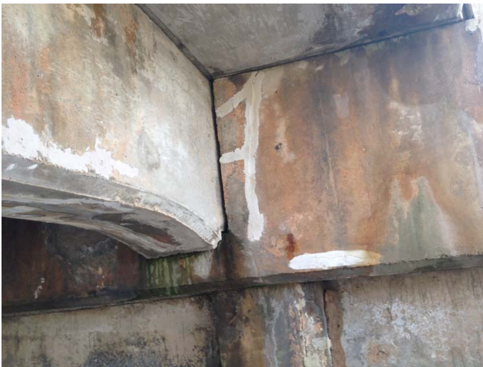
Figure 15: Cap Cracks Island Drive Structure
