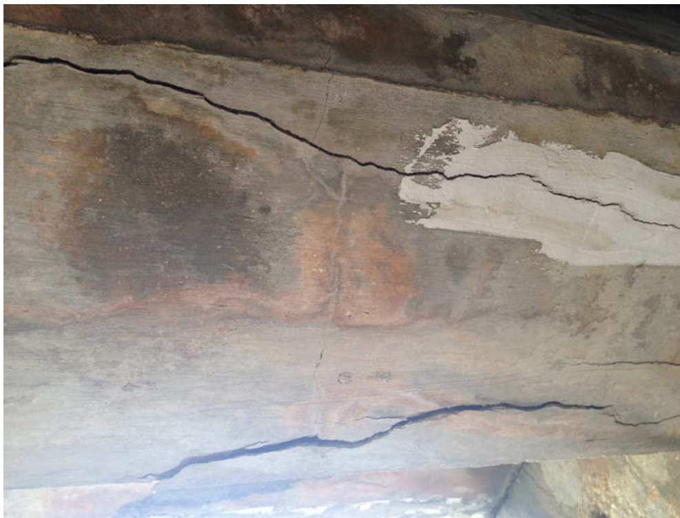
Figure 21: Beam Cracking Island Drive Structure
