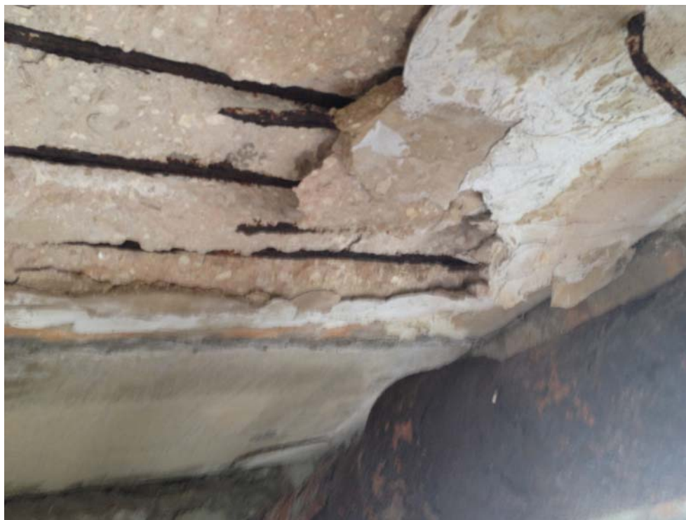
Figure 40: Deck Spalling & Reinforcing Corrosion Grand Bahama Lane Structure
