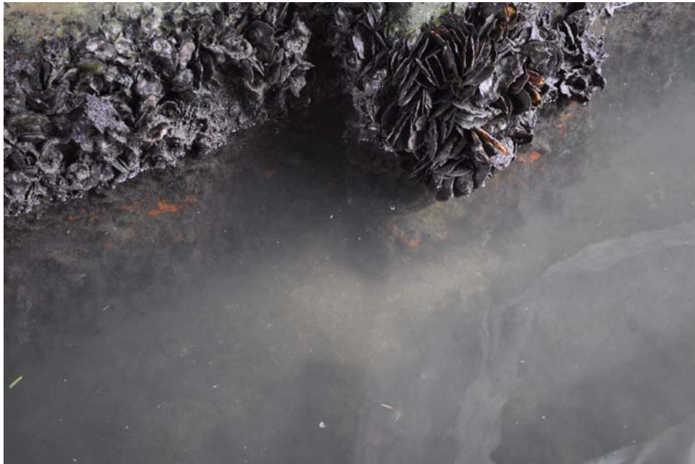
Figure 32: Retained Material Leak Island Drive Structure
