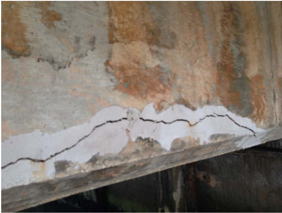
Figure 26: Beam Cracking Island Drive Structure
