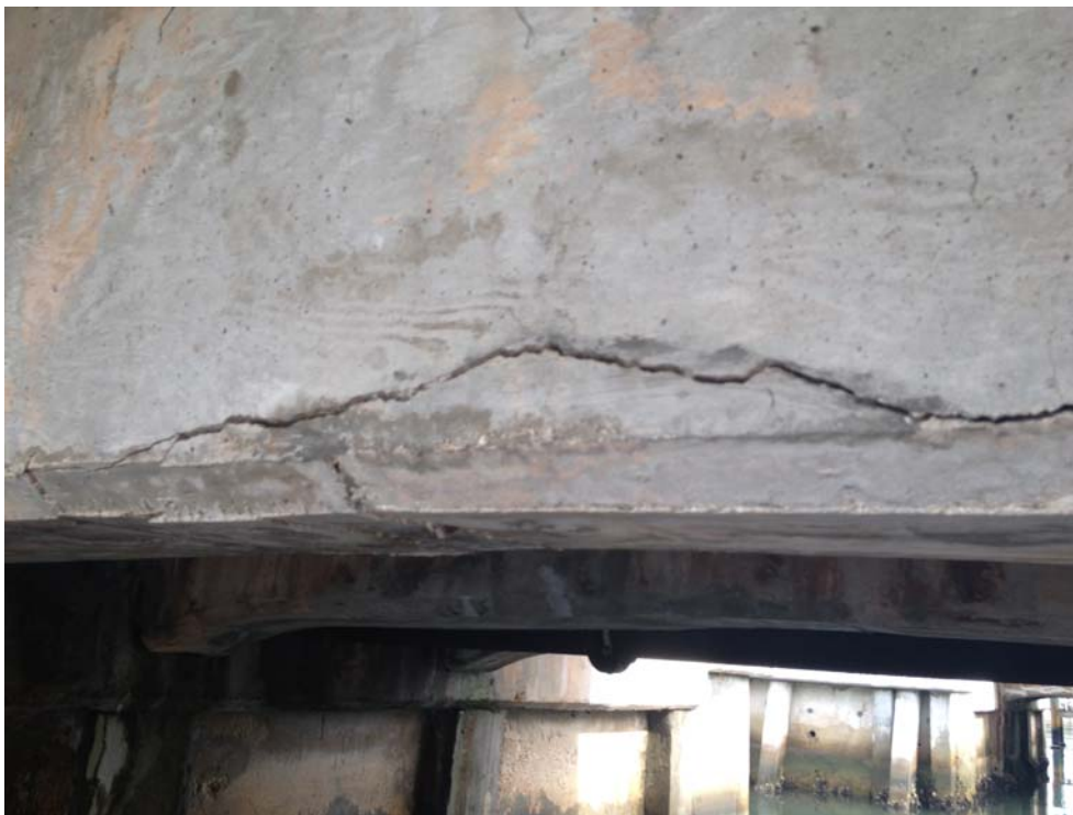
Figure 25: Beam Cracking Island Drive Structure
