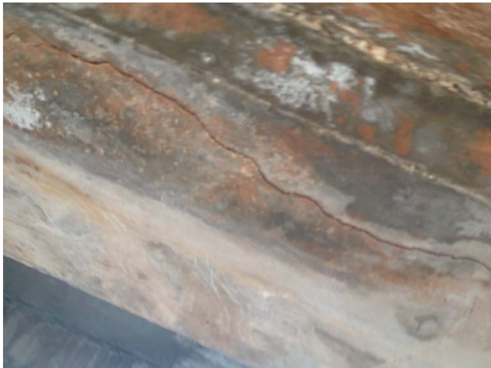
Figure 19: Beam Cracking Island Drive Structure
