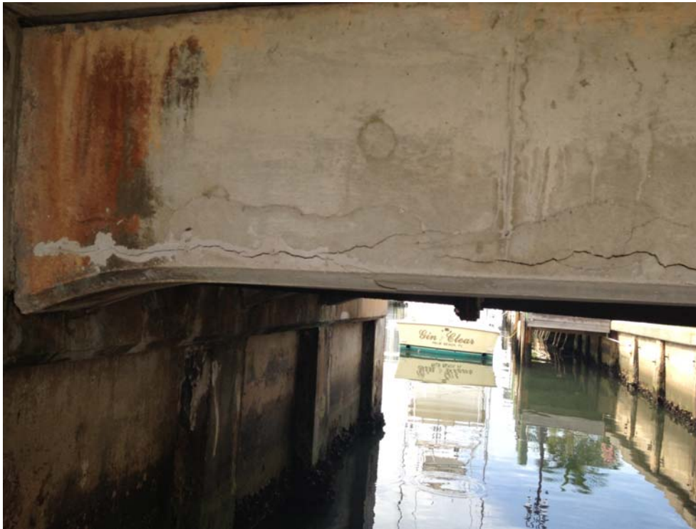
Figure 30: Beam Cracking Island Drive Structure
