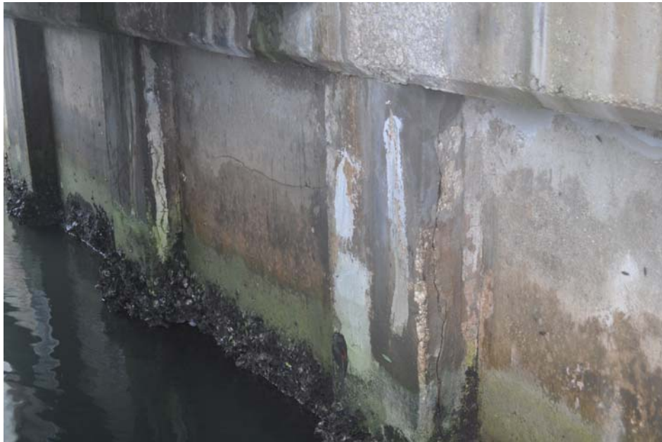
Figure 12: Pile Cracking Island Drive Structure
