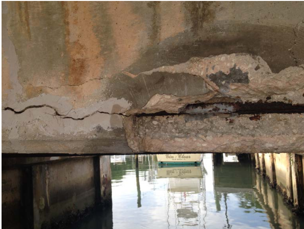
Figure 28: Concrete Spall & Reinforcing Corrosion Island Drive Structure
