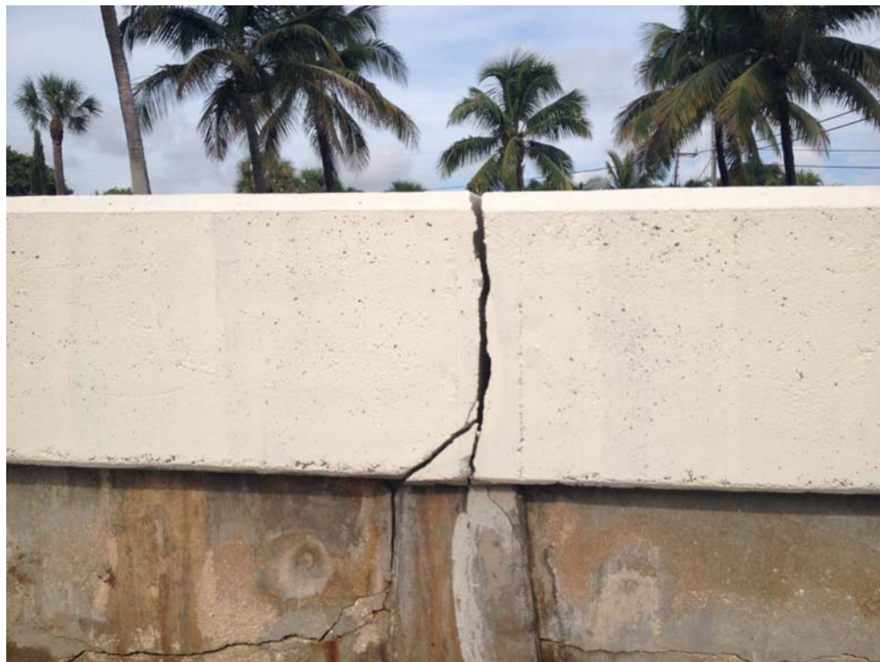
Figure 35: Bulkhead Cap Cracking Island Drive Structures
