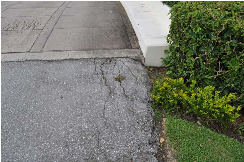
Figure 42: Asphalt Settlement Grand Bahama Lane Structure
