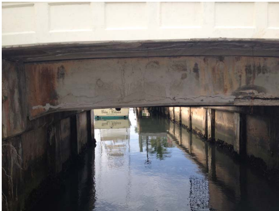
Figure 27: Concrete Spall & Beam Cracking Island Drive Structure
