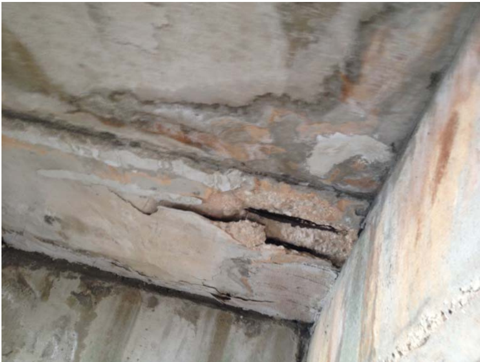
Figure 39: Deck Spalling & Reinforcing Corrosion Grand Bahama Lane Structure
