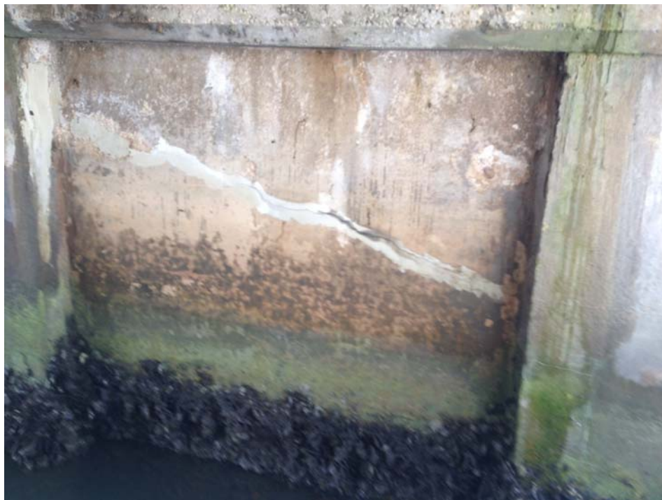
Figure 13: Sheet Panel Cracking Island Drive Structure
