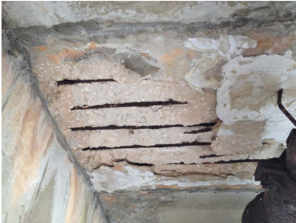
Figure 38: Deck Spalling & Reinforcing Corrosion Grand Bahama Lane Structure
