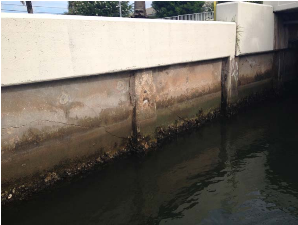
Figure 36: Sheet Panel Cracking Island Drive Structures
