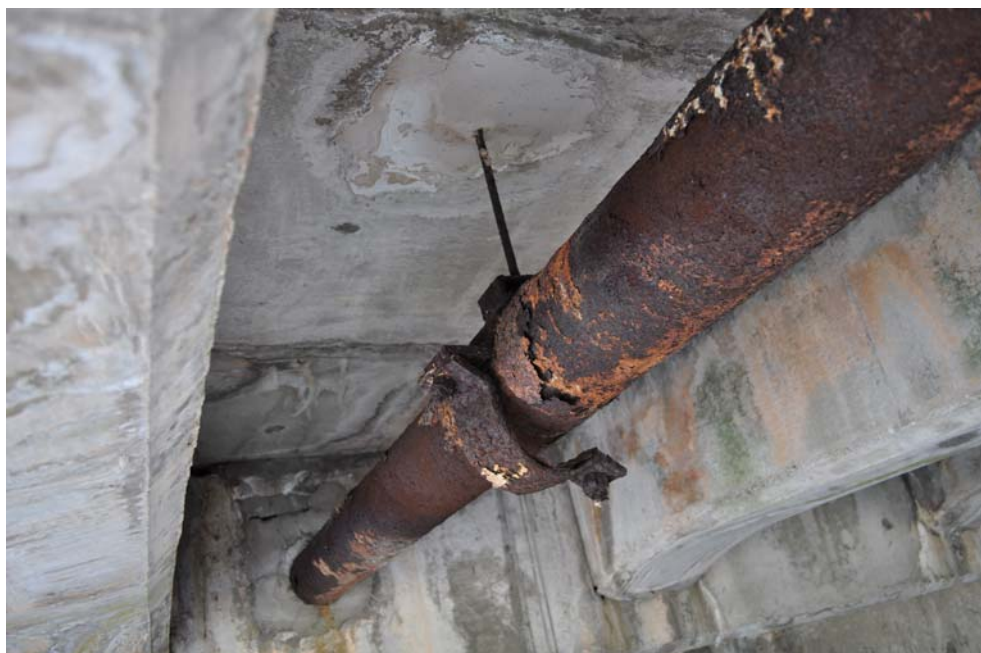
Figure 41: Pipe & Pipe Support Corrosion Grand Bahama Lane Structure
