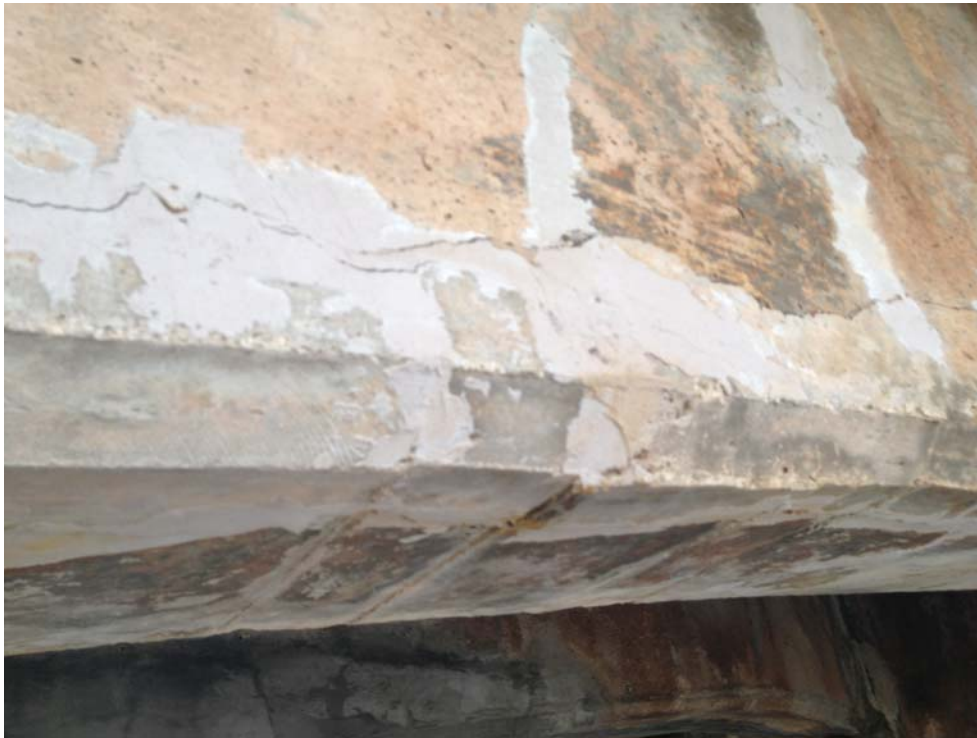
Figure 22: Beam Cracking Island Drive Structure
